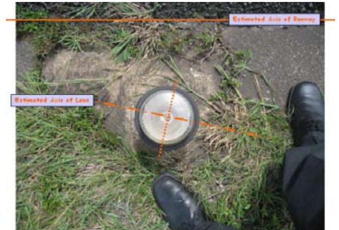
Figure 7 Example of edge light misalignment
