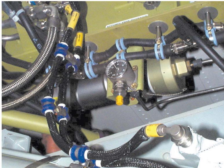
Hydraulic System 3 Accumulator Gauge Figure 13-10-6
